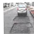
Failed utility cut
