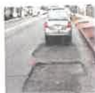
Failed utility cut
